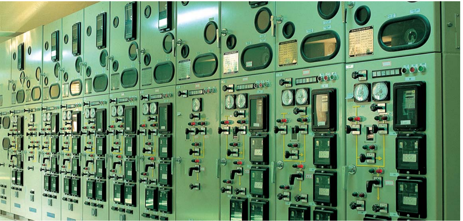
25.8kV Cubicle Type Switchgear
