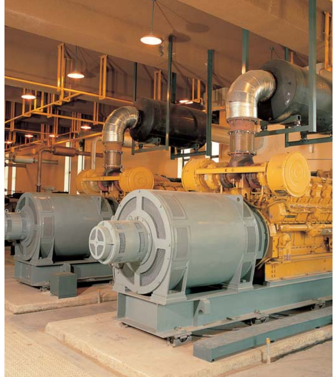
Diesel Generator in Power Plant
