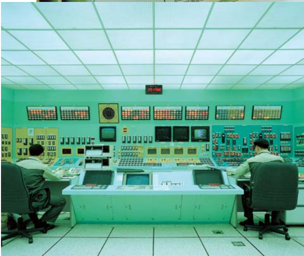
Central Control System for Nuclear Power Plant
