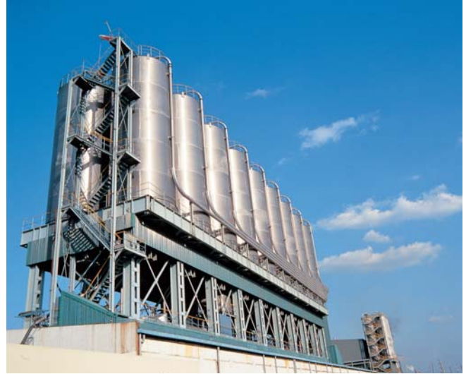
Big Silo for Polystyrene
